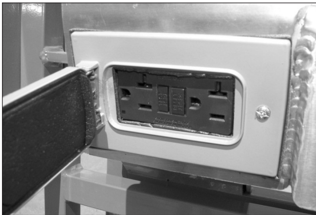
Figure 9.6 – Electrical Power Outlet
