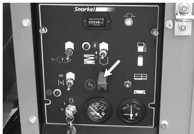
Figure 8.1 - Emergency Stop Switch at Ground Control Box
